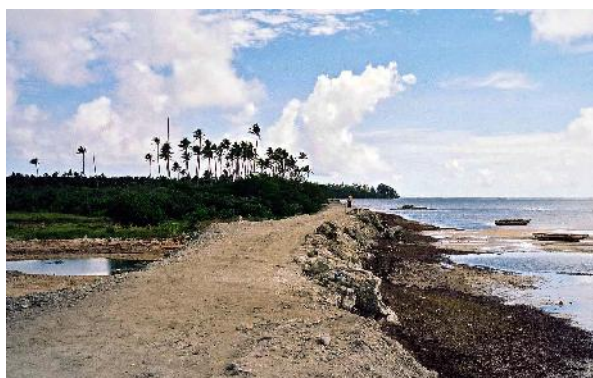
Building a sea wall on western Tongatapu, Tonga: An appropriate or inappropriate adaptation strategy? (by Ilan Kelman)
